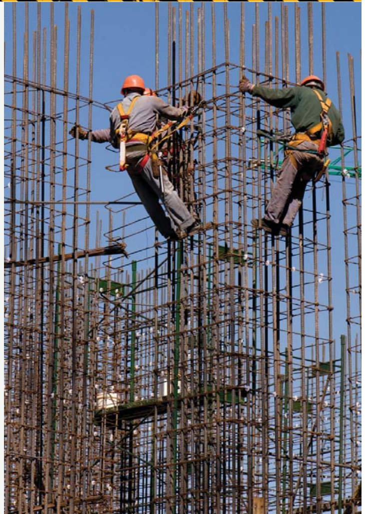
SAFETY ON HIGH: Whenever your crew members are working at elevations of six feet or higher, they need to be using the right fall protection equipment.
